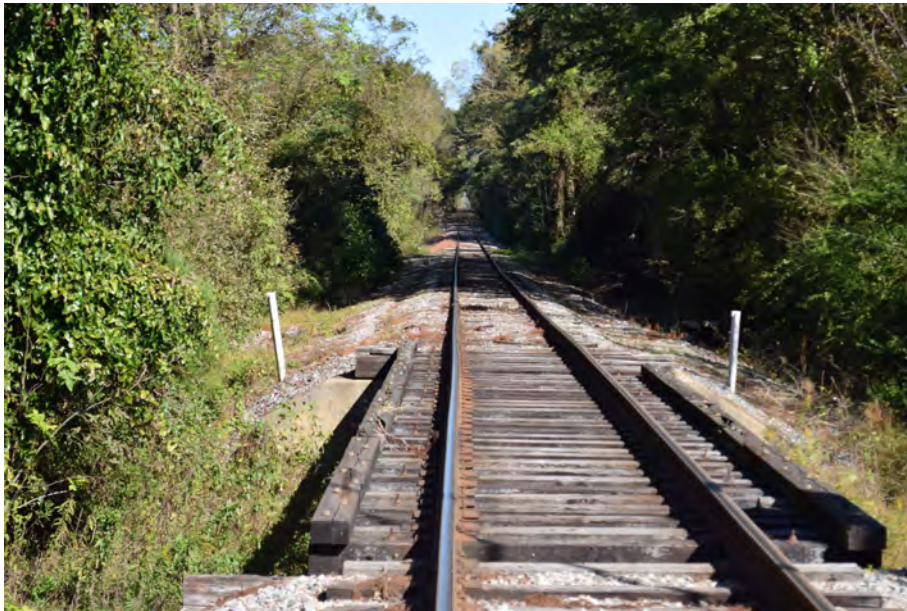
Former Washington and Plymouth Railroad (later the Norfolk Southern Railway) tracks in Bunyon, photo taken from US 264, view to the north
